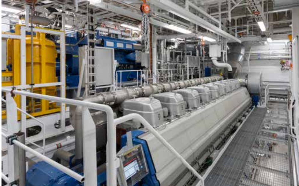
One of the four Tier-III compliant 9-cylinder Wärtsilä 46DF engines.
