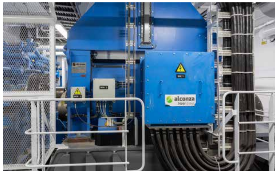
The two shaft generators provides the full power need at sea.
