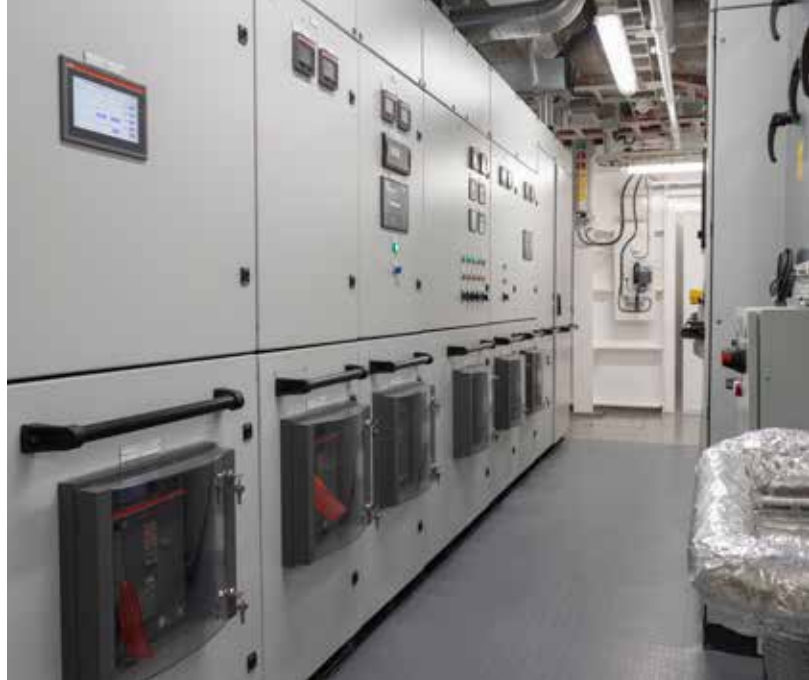
The switchboard installation is based ABB's new Ekip Link system.
